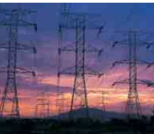
We transmit power continuously and efficiently.
