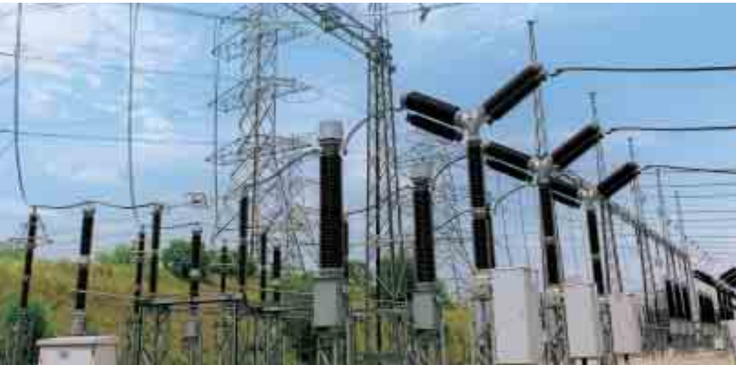
View of a main intake substation.
