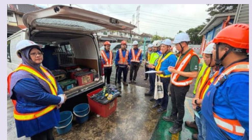
Our CPeO, Puan Feldatun Binti Sharif, observing critical substation maintenance works in Johor as part of the Group's commitment to operational safety, asset reliability and frontline engagement.
