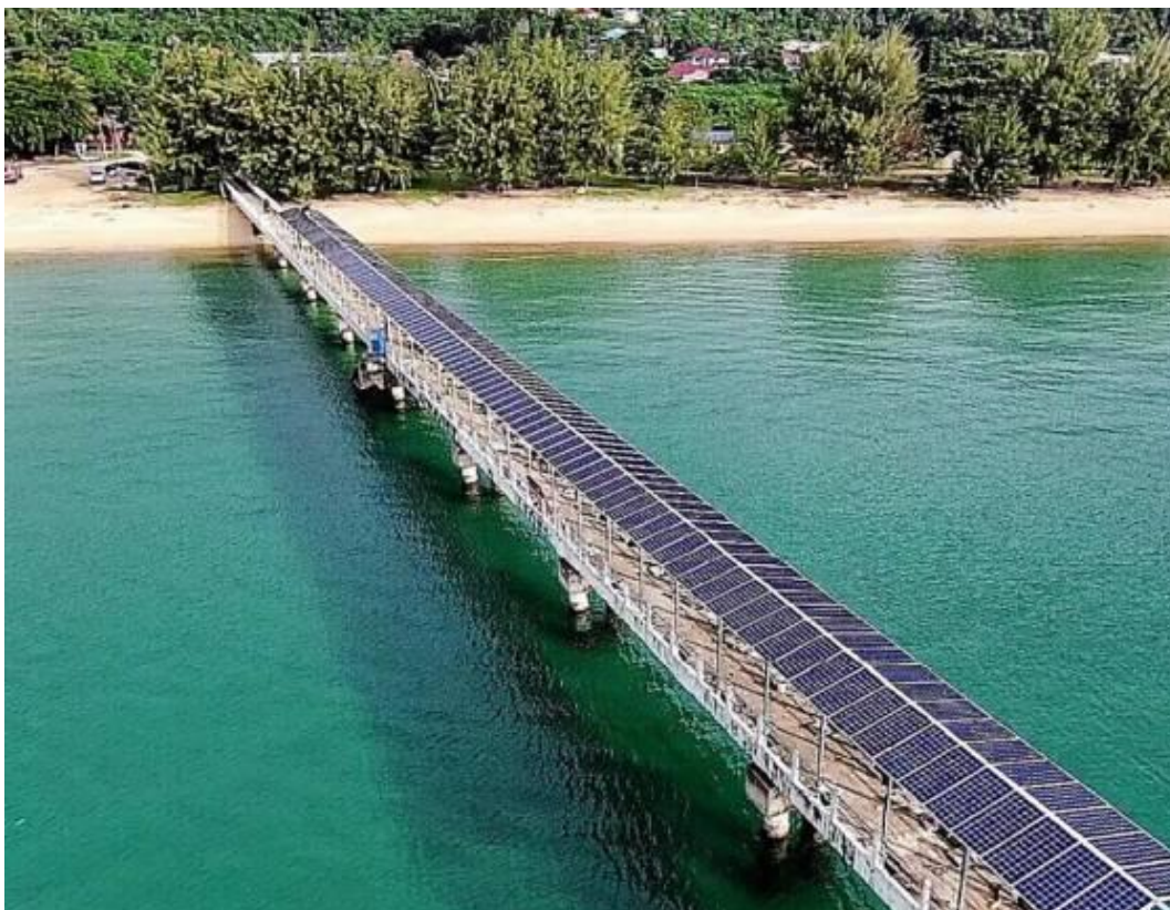
Figure 7.7: Solar PV installation at Tioman Jetty (69.39 kWp)
