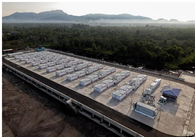
Figure 6.8: BESS Santong 100MW/400MWh
