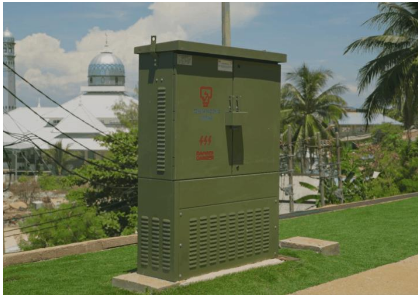
Figure 2.54: Online Feeder Pillar (OFP)
