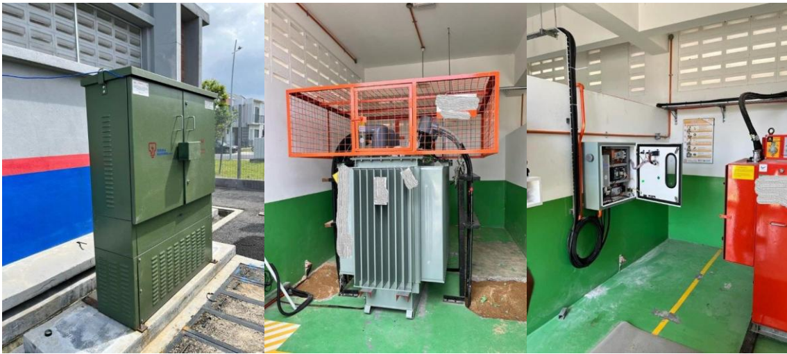
Figure 6.21: Online Feeder Pillar, Voltage Regulated Distribution Transformer & DIS
