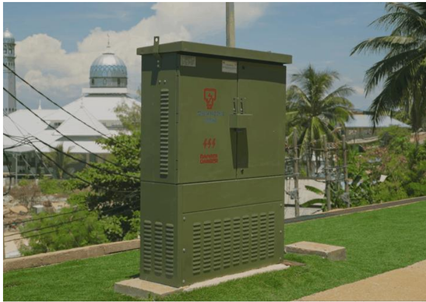
Figure 1.9: Online Feeder Pillar (OFP)
