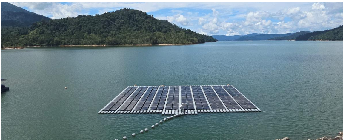
Figure 7.9: Full view of the floating solar pilot project at Kenyir Dam
