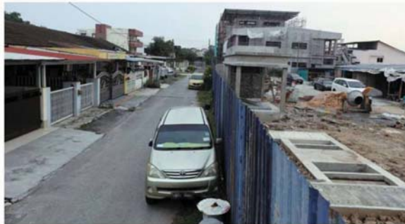
A TNB substation, rubbish disposal area and water tanks are being built opposite a row of houses along Lorong Mempelam in Klang. — Photos: KK SHAM/The Star
