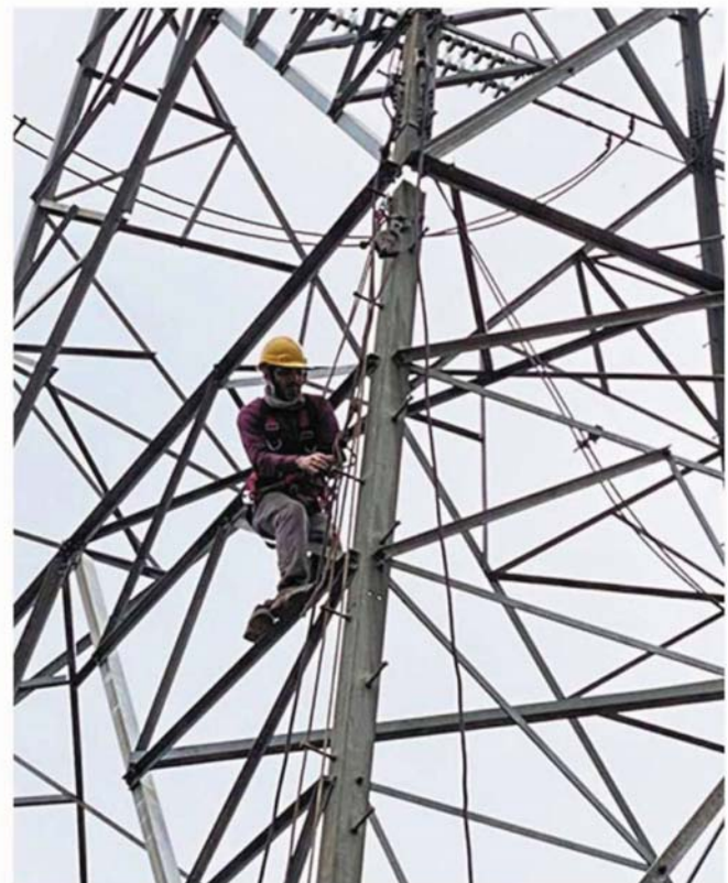
Holding things together: An SESB worker installing anchors to hold the broken metal together.
