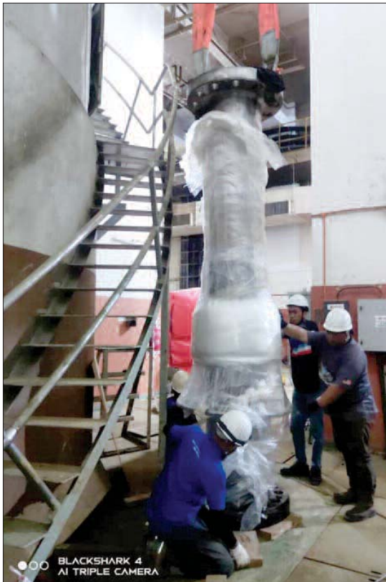
The Unit 3 turbine to be installed soon.
