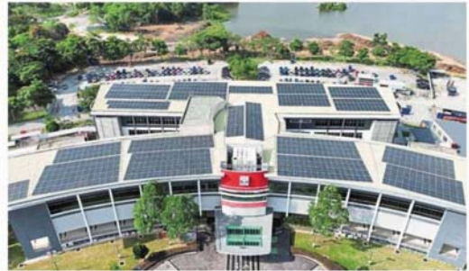
The PV system installed at the MPSepang building roof is expected to save RM105,422 in the first year of the system installation contract.
