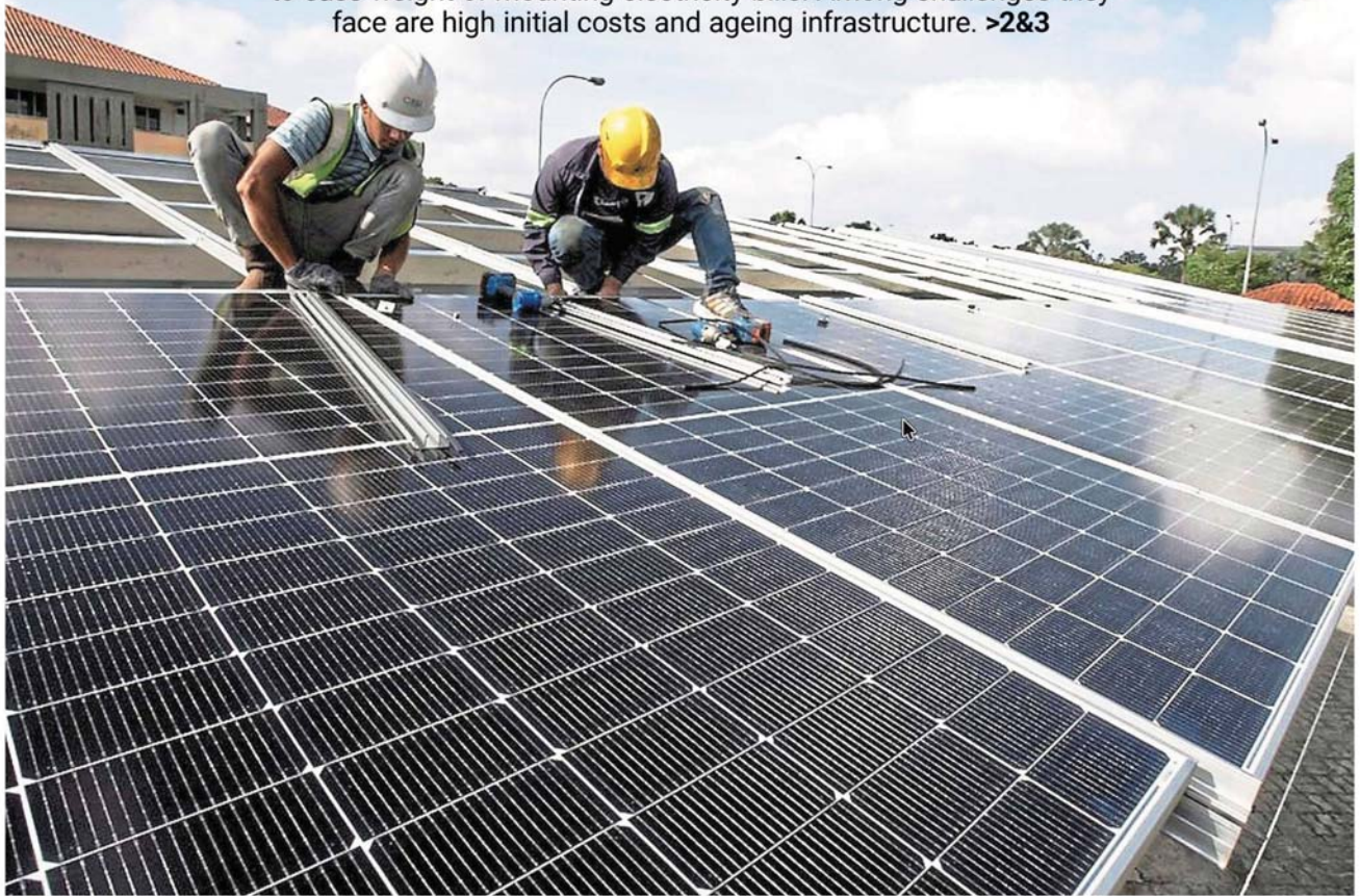
Powering on: Workers installing solar panels on the roof of SJK(C) Kuo Kuang 2 in Johor Baru. The effort is part of a RM500,000 project funded by the school's parent-teacher association and charity events, to curb high electricity bills. — Courtesy of SJK(C) Kuo Kuang 2
