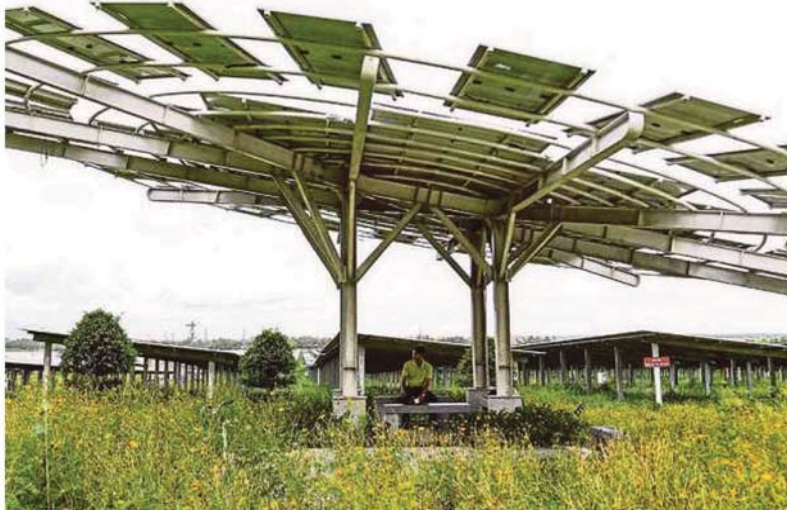
Solar power usage is increasing in Vietnam to meet climate targets, and Malaysia should be doing the same. AFP PIC
