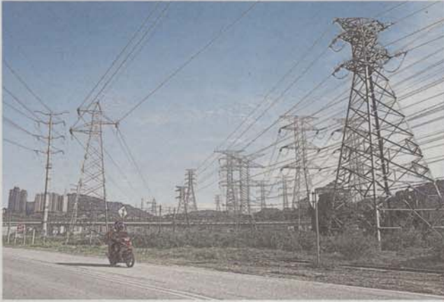
As more RE projects come online, the challenge will be ensuring that new generation capacity can be integrated into the grid without creating bottlenecks
