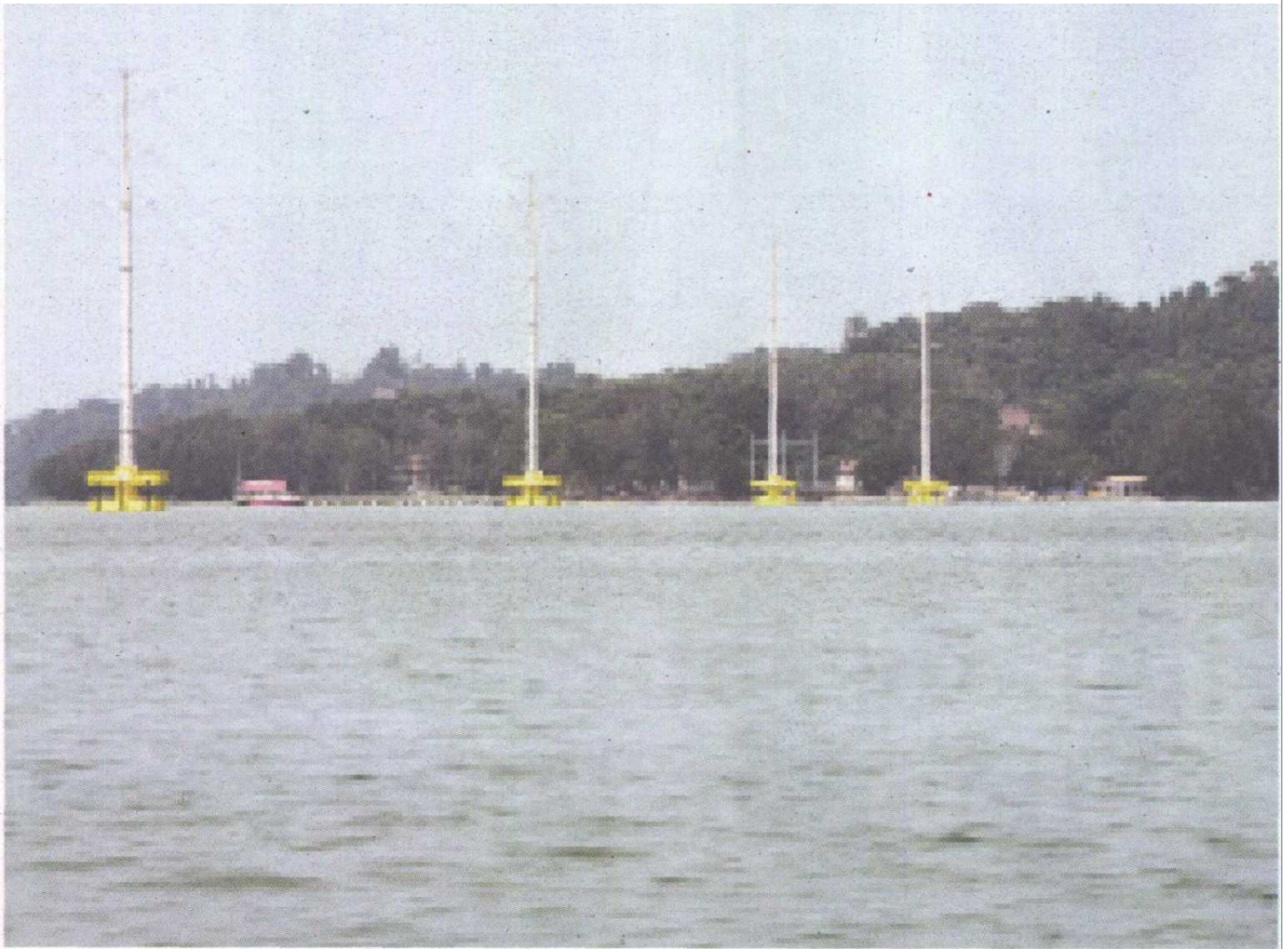
Some of the 12 monopole towers cross a 4.2km stretch of the Straits of Malacca to Pulau Besar.
