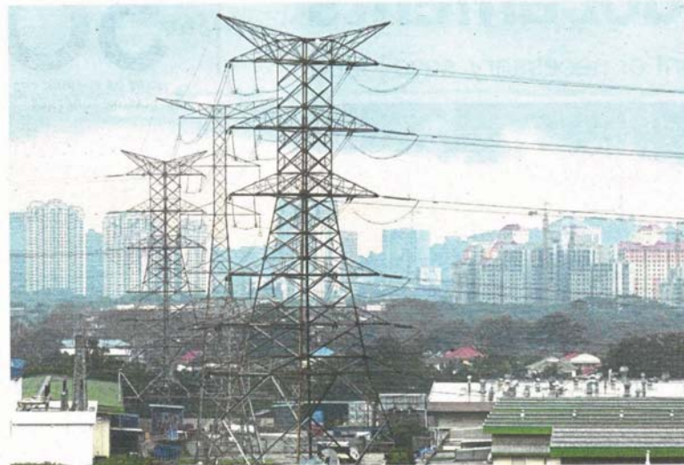
The electricity grid of the future will not be just wires and cables carrying electricity from one place to another.
