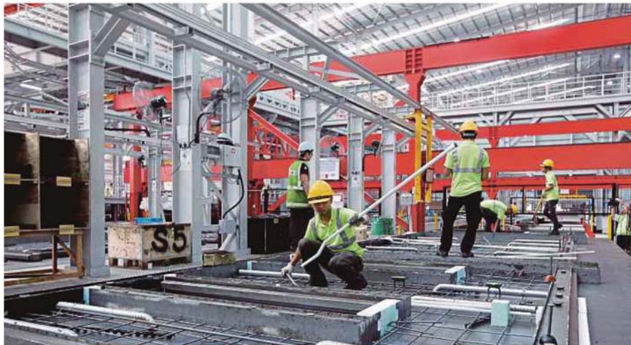
Workers carrying out maintenance work on Gamuda Bhd's industrialised building system plant in Banting, Selangor. FILE PIC
