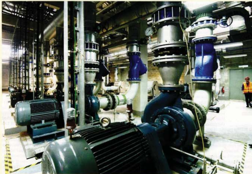
High-efficiency chillers are used in district cooling plants to minimise energy consumption while maximising cooling capacity
