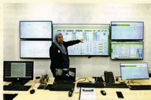
The control room is responsible for remote monitoring of operations, controlling machine performance and making critical decisions
