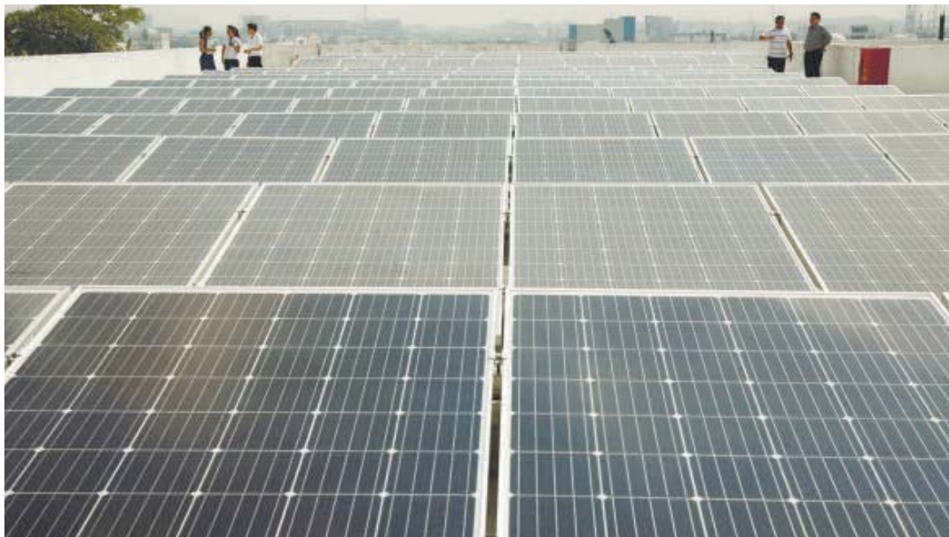
A view of JTC and Sun Electric's SolarRoof project in Singapore. - REUTERS/PIC
