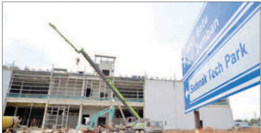
Sedenak Tech Park in Johor's Kulai district will be the biggest data centre in Malaysia. (CNA)
