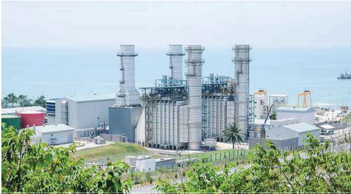
The Telok Gong Power Station 2 is a combined cycle gas turbine power plant with a capacity of 705 megawatts.
