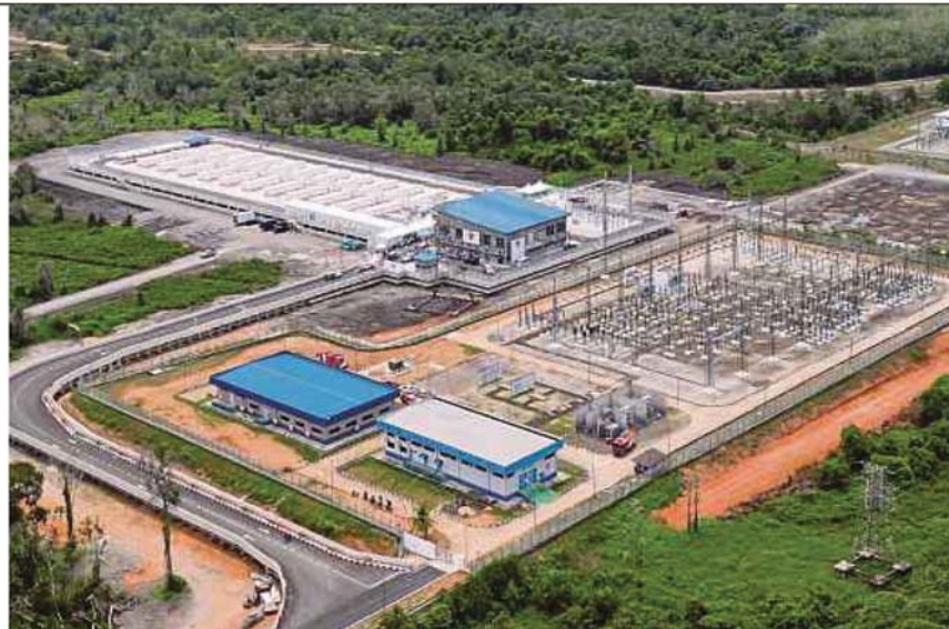
Tenaga Nasional Bhd's Santong battery energy storage system has a capacity of 100 megawatt/400 megawatt per hour. BERNAMA PIC
