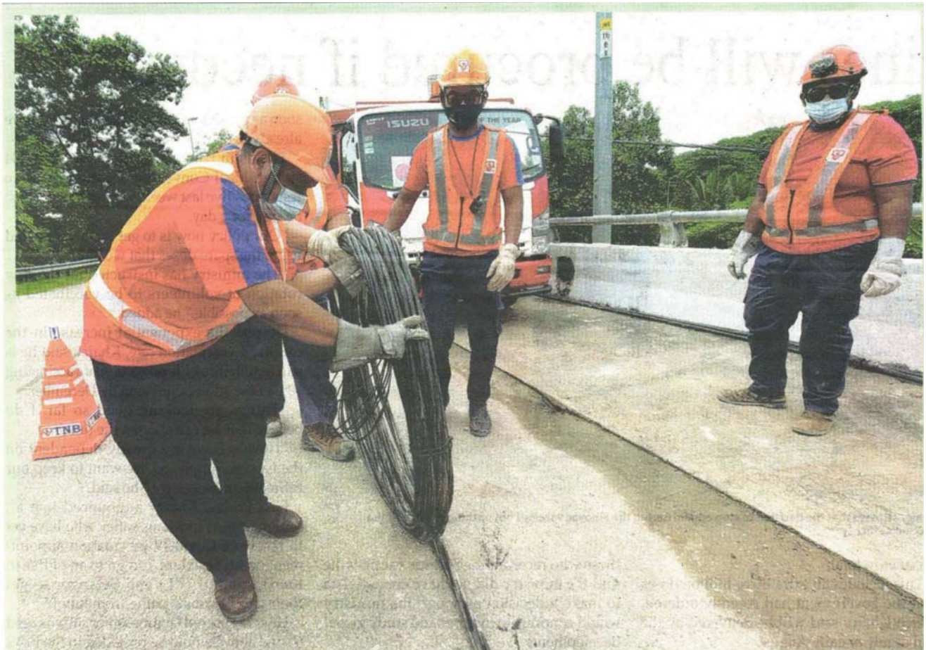
DELIVERING BEST SERVICE: Employees of Tenaga Nasional Bhd (TNB) laying out cables before starting recovery work at the Kampung Rengai electrical substation in Kuala Lipis, Pahang. They are some of TNB's frontline technical staff who continue to work hard to ensure that electricity supply remains stable and reliable for its 9.5m customers. TNB is committed to continue delivering the best service throughout the implementation of the current Movement Control Order.
