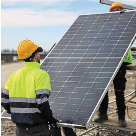
Workers installing a solar panel in Trino, Italy, last month. Clean energy is one of the great hopes for healing a polluted planet. — Reuters
