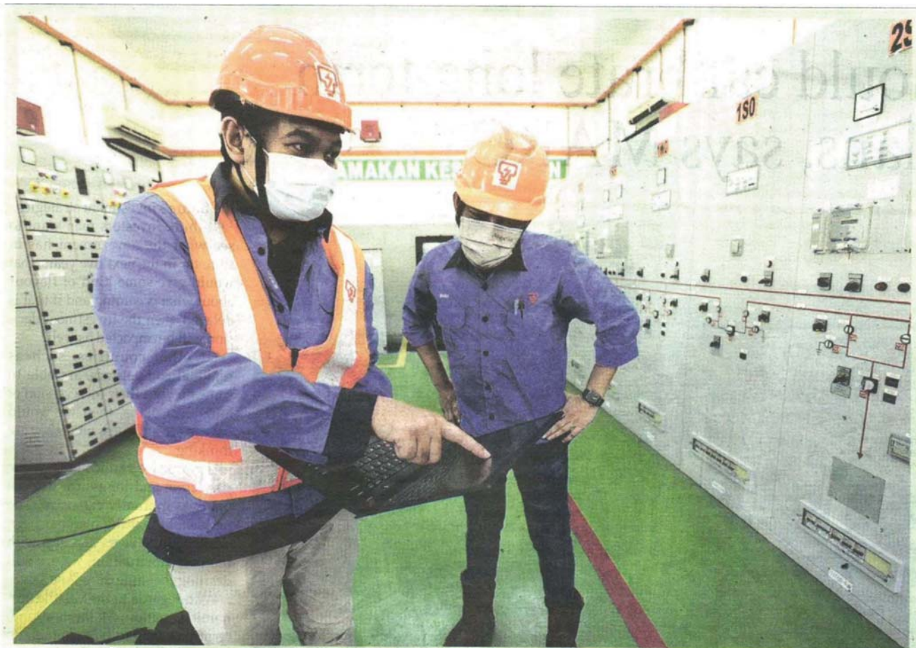
STABLE SUPPLY: Tenaga Nasional Bhd (TNB) Selangor technicians Mohd Hafiz Fikri Arazmi (left) and Mohd Shahril Nor Shah inspecting the Main Switching Station of Universiti Teknologi MARA (UiTM) Puncak Alam in Shah Alam, which supplies electricity to the UiTM Puncak Alam Mega Vaccination Centre (PPV). TNB has always been committed to prioritising the stability and reliability of electricity supply to hospitals, vaccine storage centres (PSV) and vaccination centres, as well as temporary police and military security posts. Since the Movement Control Order 1.0 in March last year, TNB has contributed more than RM33m towards this purpose and is now focusing on ensuring electricity supply at more than 40 PSVs and more than 400 PPVs remains stable.
