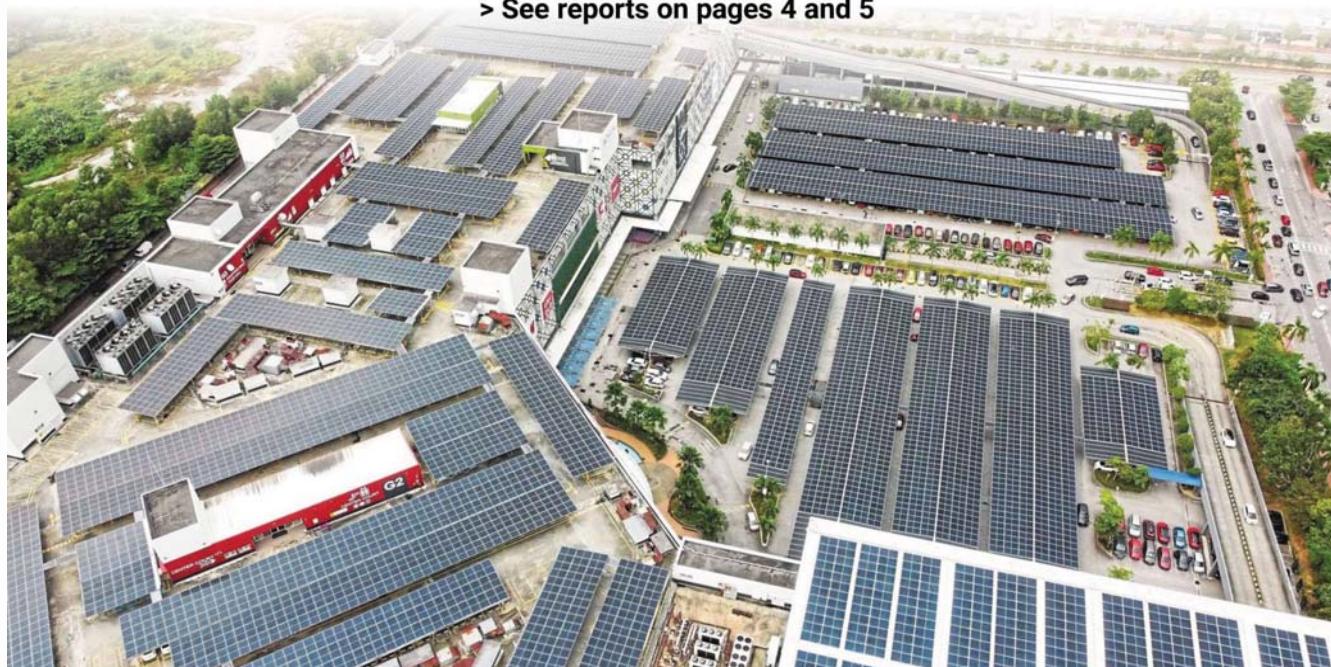
Sun power: Solar panels installed on the rooftop of AEON Mall Shah Alam in Selangor. Solar is emerging as the primary driver of renewable energy growth in Malaysia. — IZZRAFIQ ALIAS/The Star
