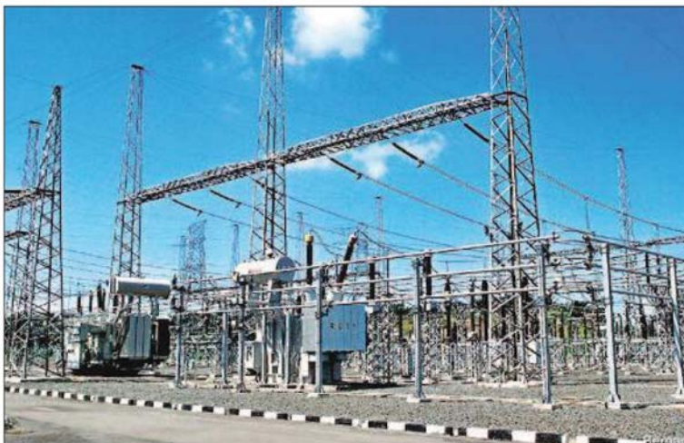
A view of an electrical substation and high-voltage transmission infrastructure.
