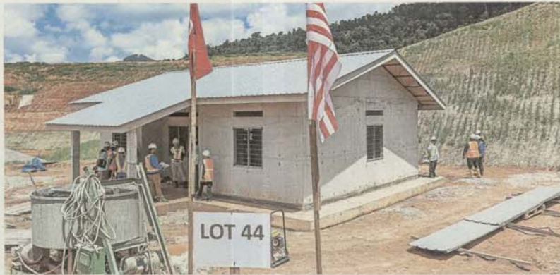
New settlements with improved facilities are being built, including 93 housing units for Pos Pulat and Kuala Wias villagers, and 191 units for Pos Tohoi residents
