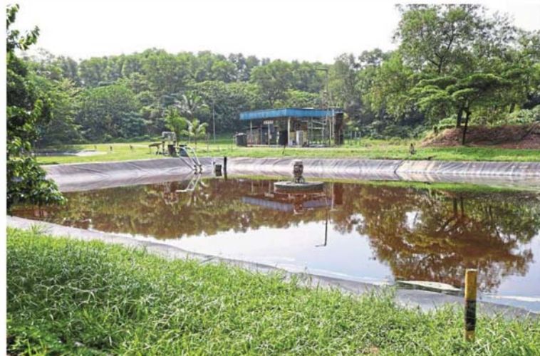
A leachate treatment plant at the Worldwide Landfills Park, Air Hitam, Puchong. — Photos: GRACE CHEN and LEONG WAI YEE/The Star
