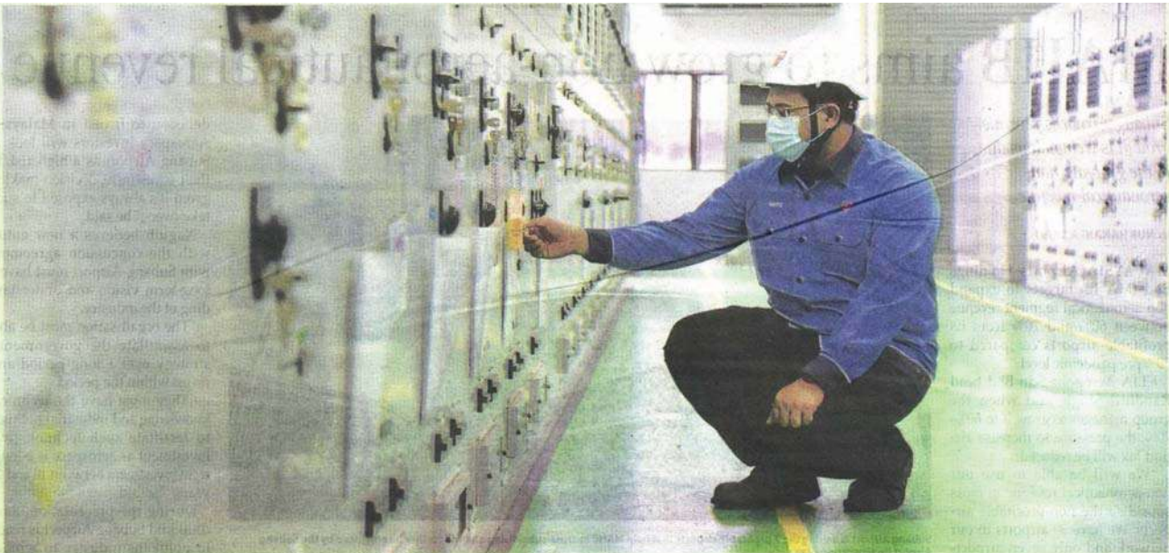
ELECTRIFYING THE NATION: Selangor Grid Maintenance Senior Engineer (Lines and Cables) Mohd Hafiz Jamil carefully carrying out switch maintenance duties at the Main Inlet Substation in Bukit Beruntung, Selangor. Tenaga Nasional Bhd continues to actively support the country's efforts in curbing the current Covid-19 crisis by ensuring the best services as well as continuous and stable electricity supply at critical locations such as hospitals, vaccination centres and vaccine storage centres, especially during the stricter implementation of the Full Movement Control Order or FMCO.
