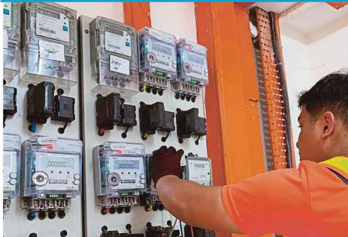
FGV Prodata Systems Sdn Bhd has been given an extension to expedite the installation and support systems for Tenaga Nasional Bhd's smart meter project until March next year. FILE PIC
