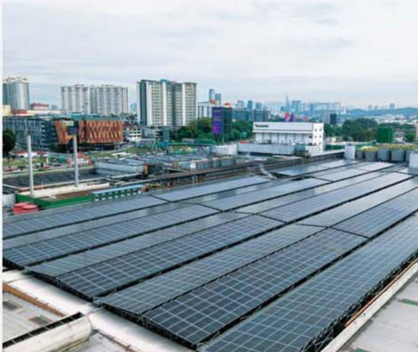
3,500 mono-PERC solar panels installed on Sungai Way brewery roof
