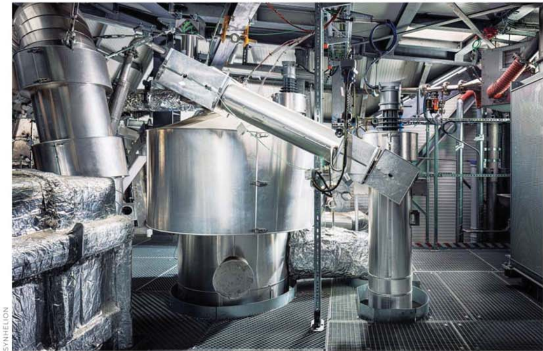
Synhelion's proprietary thermal energy storage and thermochemical reactor at plant DAWN
