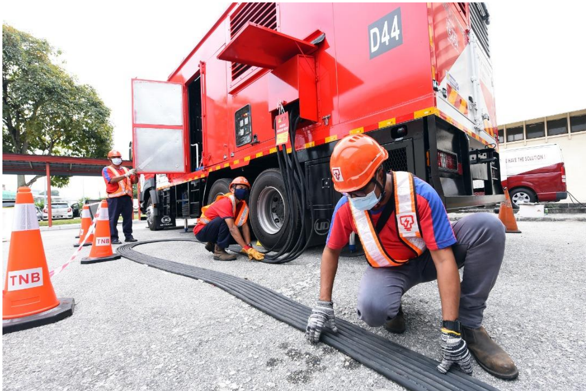
TNB technical team carrying out temporary shutdown work for maintenance and installation of a remote automation supply system, Remote Terminal Unit (RTU) at a hospital in Selangor on 20 February 2021.
