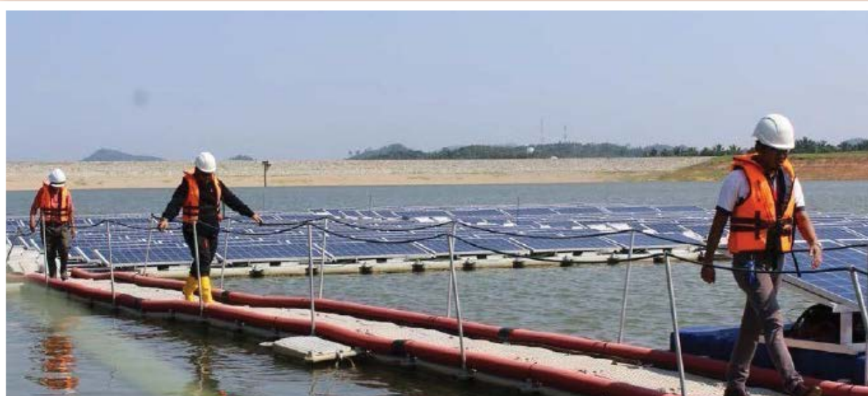
Country's first floating solar project at Sungai Labu Water Treatment Plant, Sepang, Selangor.
